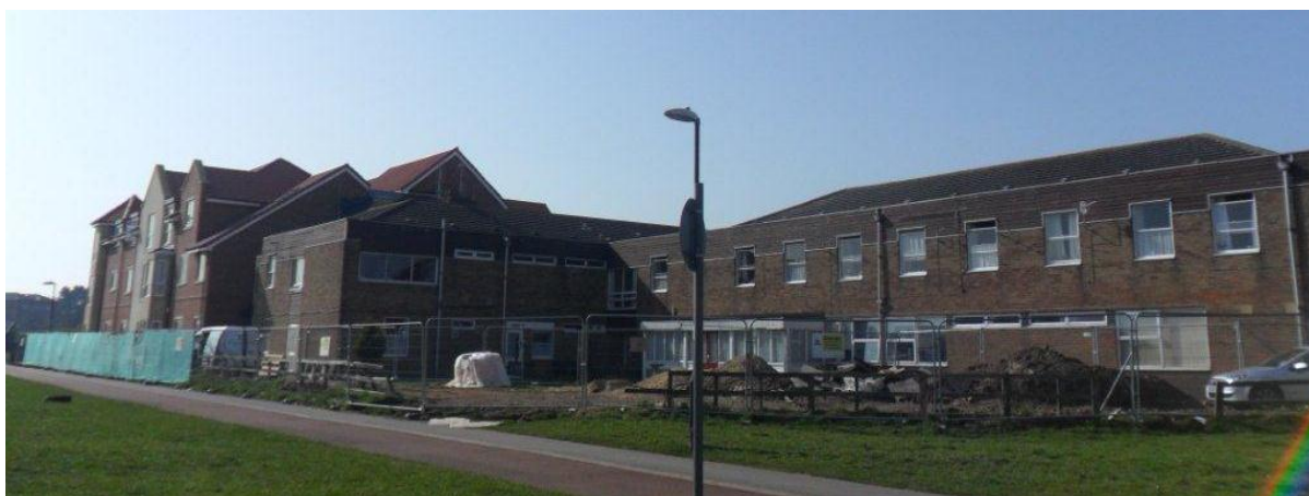
Cherry Garth Elderly Persons' Home transforming in a two-phase build process into Meadowfields Extra Care
